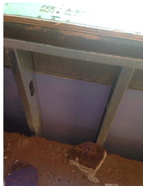
Figure 3 Shows 5 inch gap
