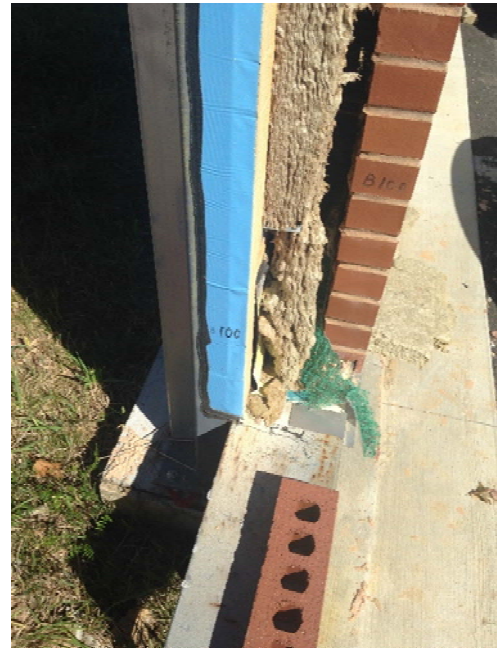
Figure 5 Brick hangover on lintel
